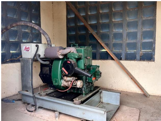
Diesel Generator for pumping water
