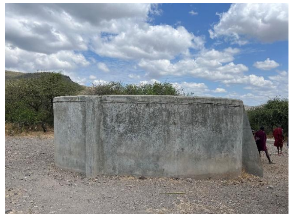
50 cubic metres concrete water tank
