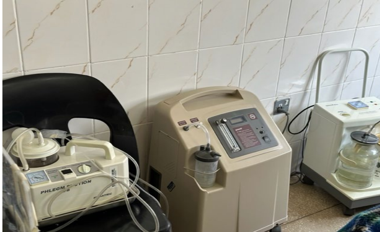
Pictured above are suction units and an oxygen concentrator that were nonfunctional.
