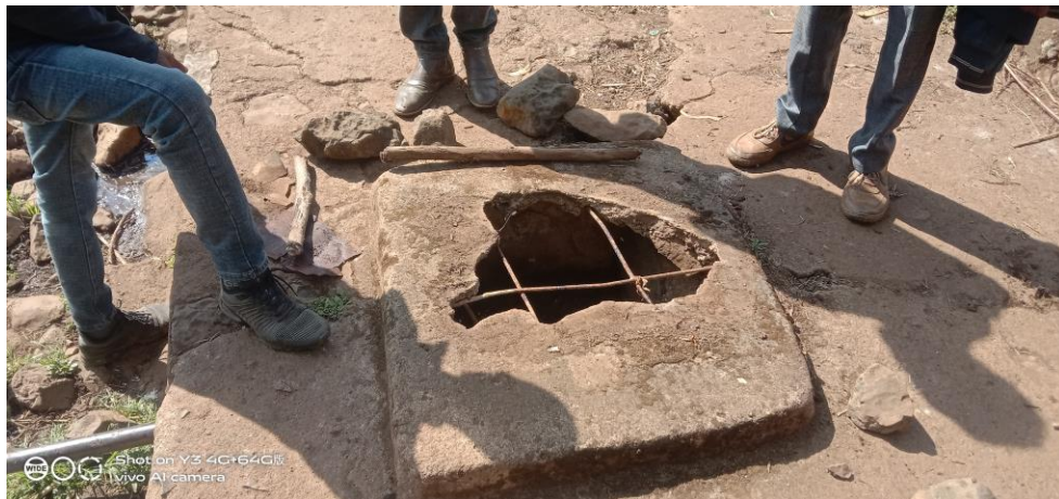
b) Damaged construction & flooding and any precipitation runs into the collection chamber
