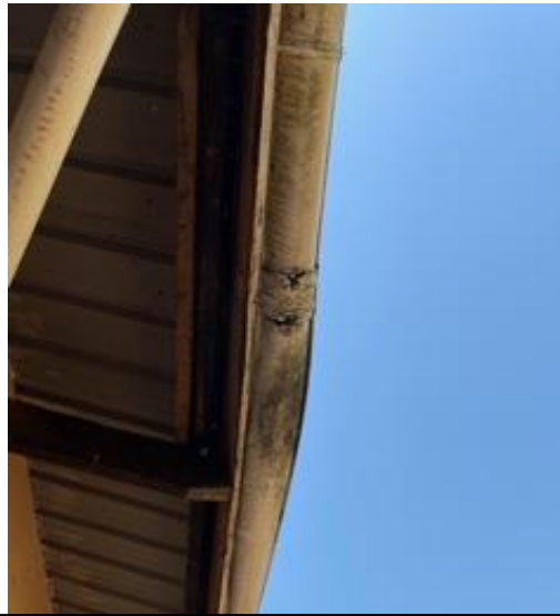
The rain water harvesting gutters are dilapidated
