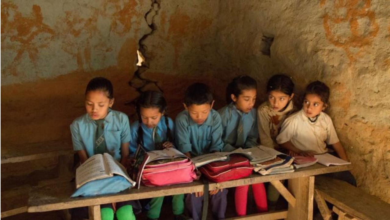
Students attending school in earthquake damaged classroom.
